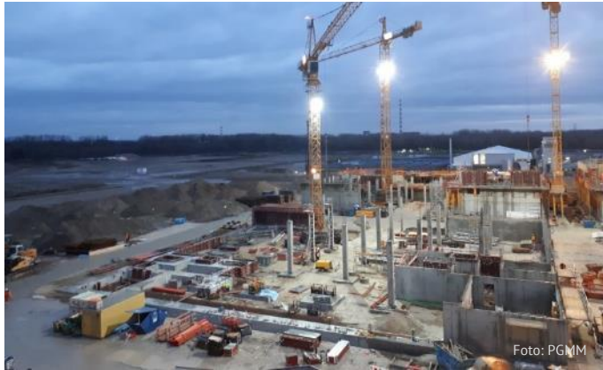
Audi AG Ingolstadt Central power unit and infrastructure Innovationscampus
